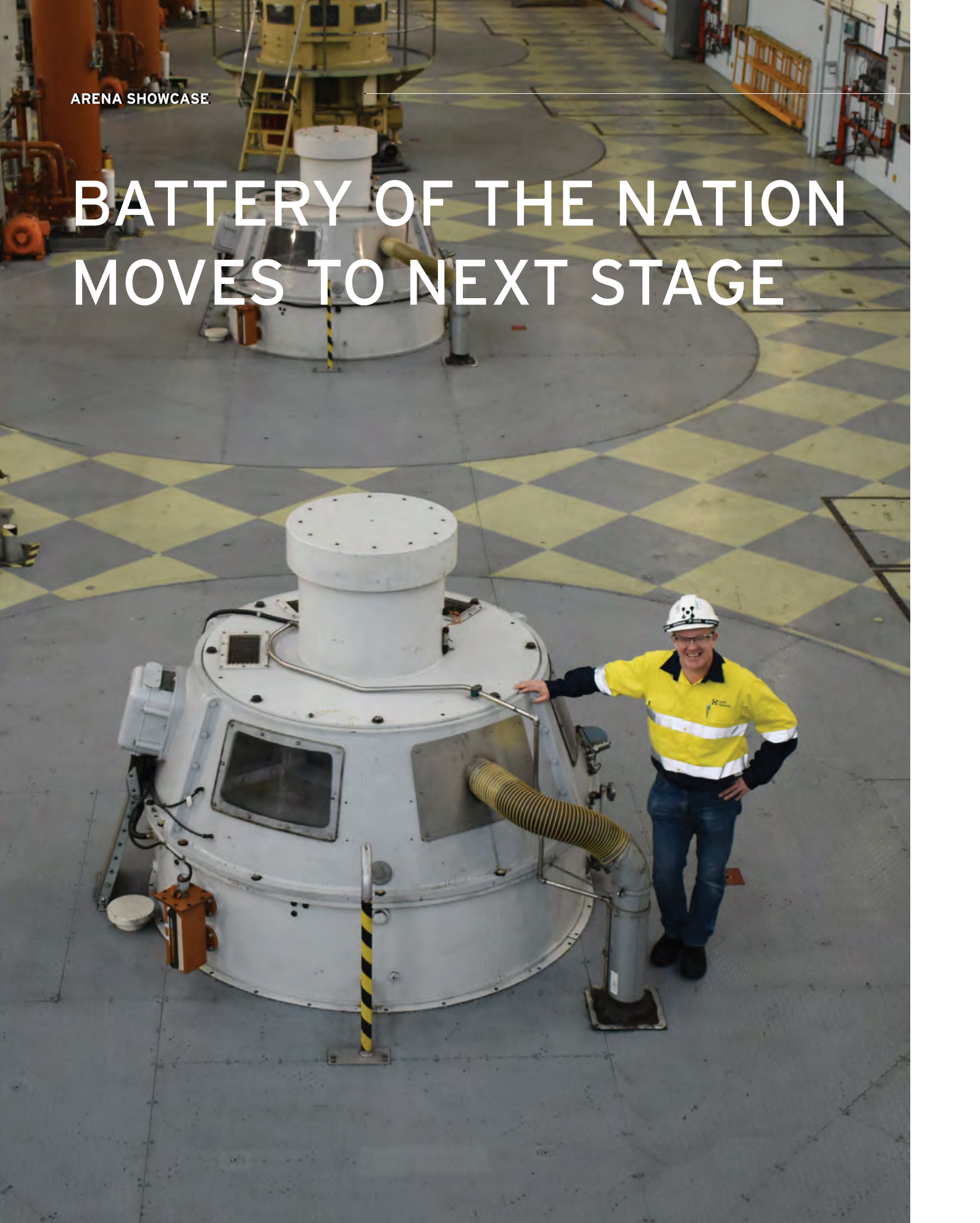
The floor of the Trevallyn power station in Launceston. Image credit: Hydro Tasmania.
